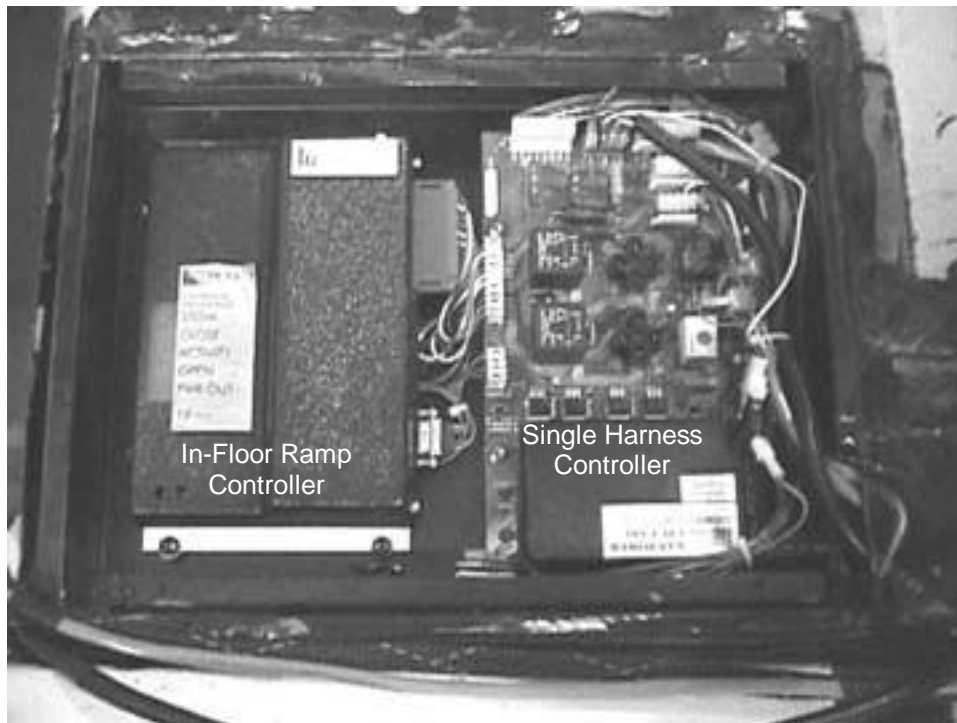
Access Panel in rear of vehicle, with carpet and cover removed.
